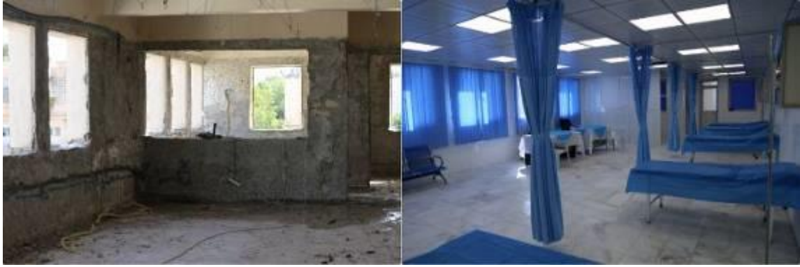
One of the damaged rooms at the Emergency Department before and after renovation.
