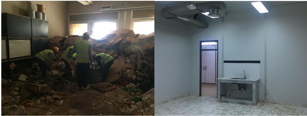
Before and after rehabilitation work at the Animal House Building in Benghazi University. ©UNDP Libya
